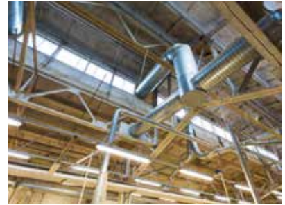
Climate control & ventilation plants
