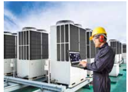
Building management systems
