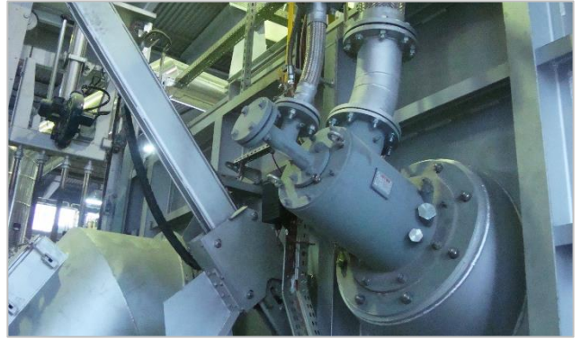
Aluminium Holding Furnaces
