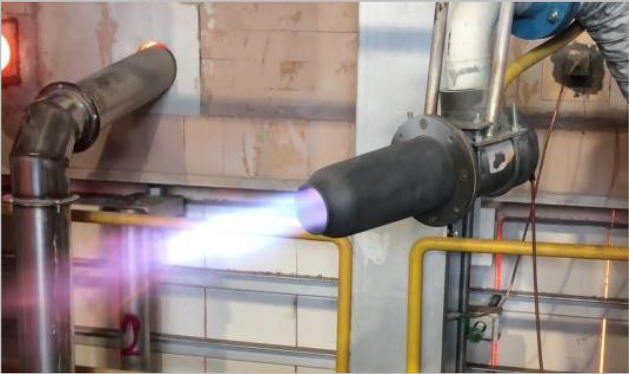
Glass Holding Furnaces
